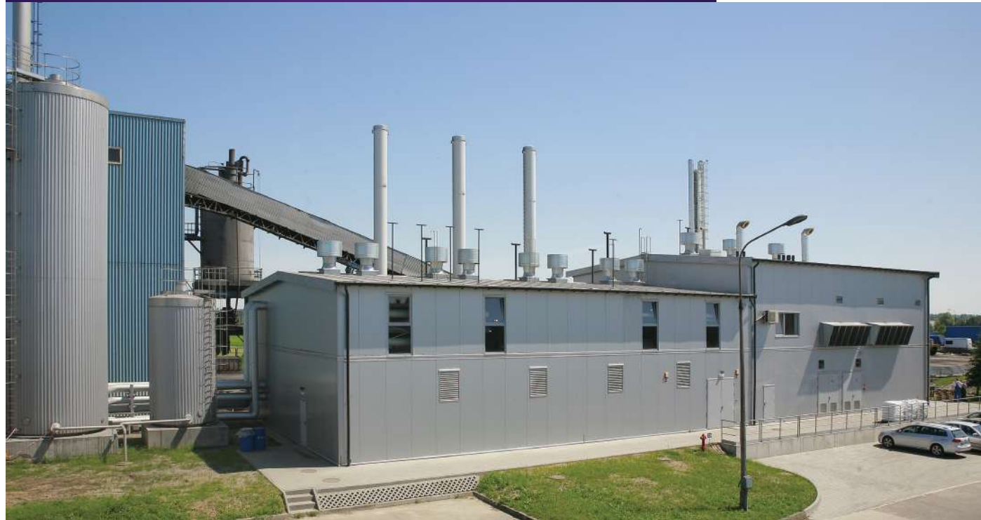
Condensation plant - Sokołowie Podlaskim - Poland.
